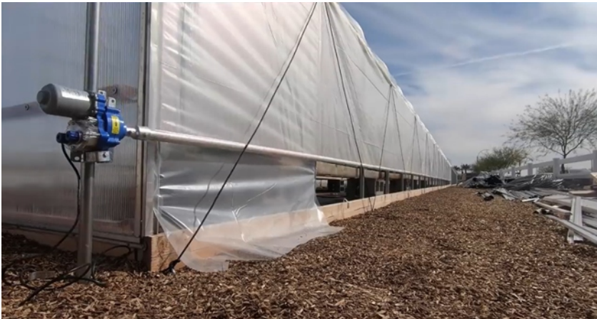
Image 63: Roller motor for a tunnel greenhouse that is equivalent to the greenhouses at Vegetable Garden de Haar
