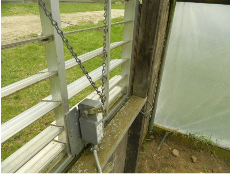
Image 45: Louvre window in greenhouse that can be opened and closed with electric control. Form of passive ventilation.
