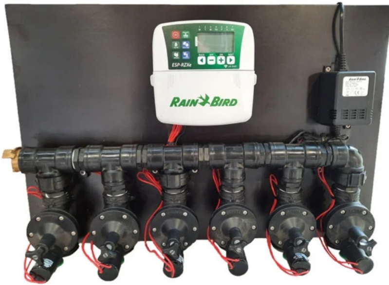
Image 68: Distributor with electric valves for irrigation
