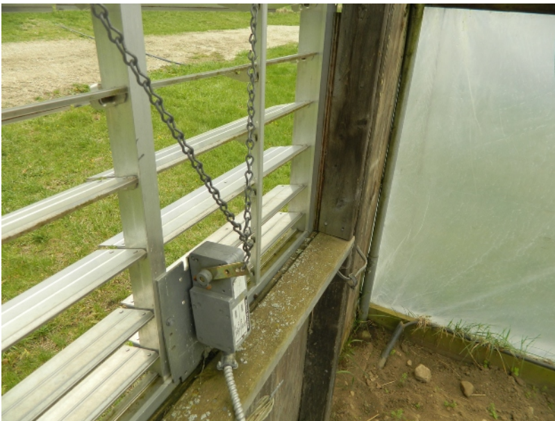
Image 61: Louvre window in greenhouse that can be opened and closed with electric controls. Form of passive ventilation.
